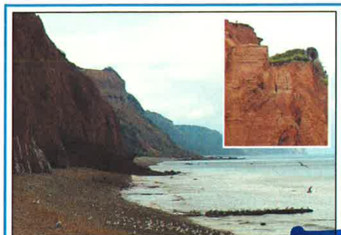
▲ Danger zone: the latest cliff fall at Pennington Point and (inset) cracks remain visible.
